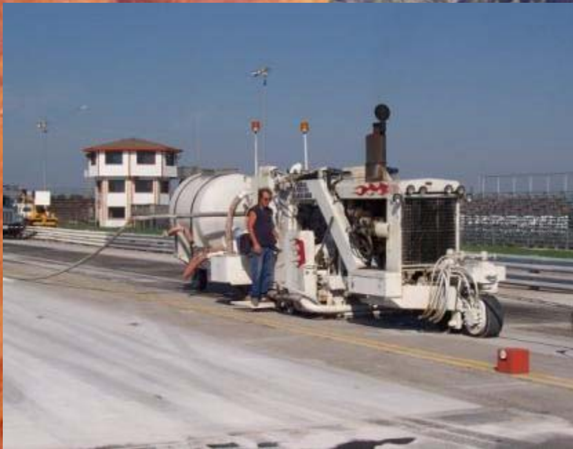
Typical Grinding Equipment
